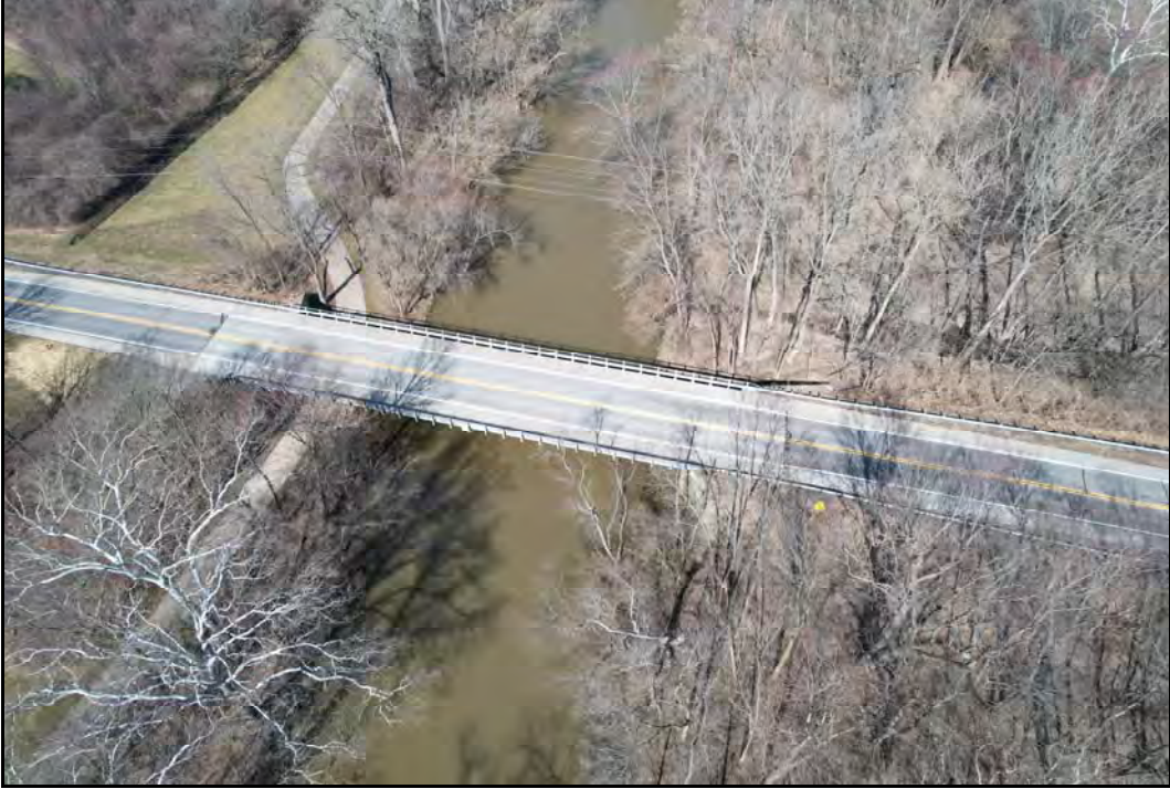
Looking north at Alum Creek bridge. Bridge is maintained by the Franklin County Engineer. Three Creeks Metro Park is on north and south side of road.
