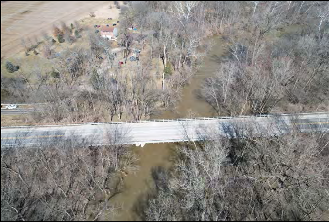
Looking north at bridge over Big Walnut Creek. Bridge is maintained by the Franklin County Engineer. Three Creeks Metro Park is on south side of road.
