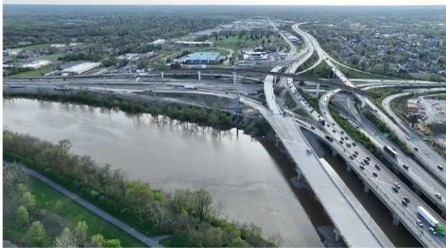
Drone views of I-70 and I-71 construction through downtown Columbus Drone views of I-70 and I-71 construction through downtown Columbus.
